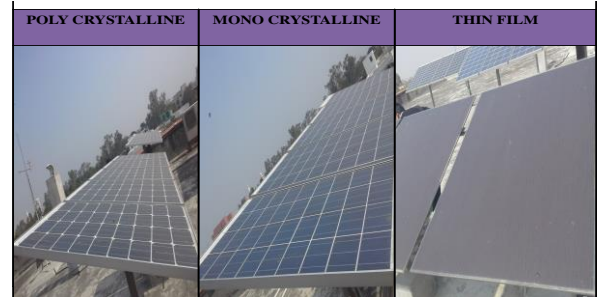
Fig. 2 PV panels installed on roof-top
