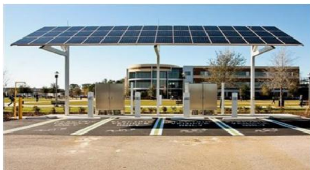
Fig.1 PV Based EV Charging Station.
