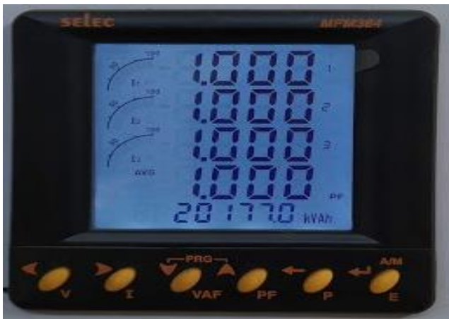
Fig. 16. Multi function energy meter shows power factor to unity on the bus.
